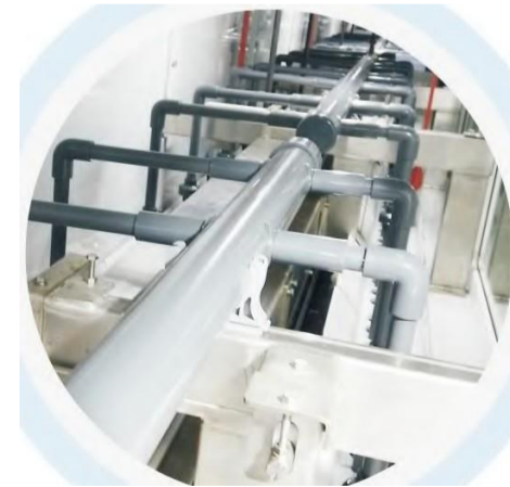
Automatic pumping device for copper plating residue
