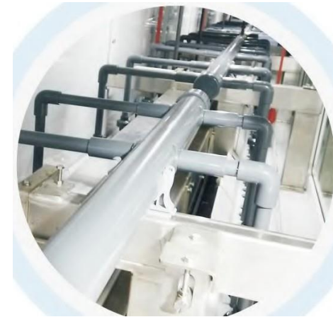
Automatic pumping device for copper plating residue
